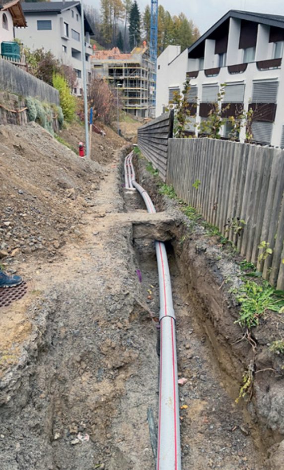
Provediment electric en in foss
